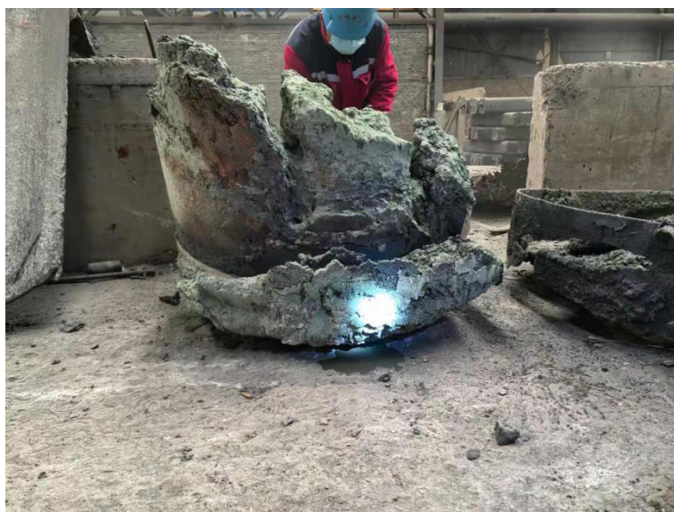
图7 拆炉后炉底残余钢块
